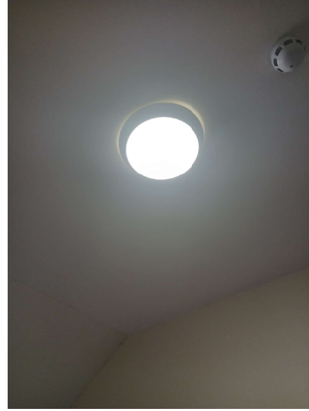
Lighting (Standard and Emergency Lights)
